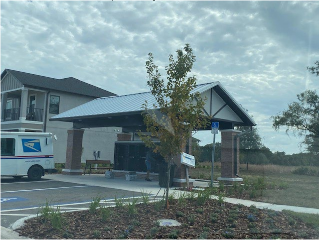
Green Briar mail kiosk almost complete. Waiting for electric.
